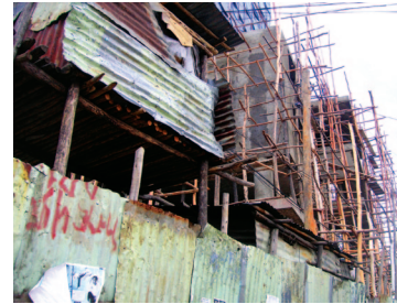
Growing cities mean growing demand for timber products to use in construction, such as this scaffolding in Yaoundé, Cameroon.
